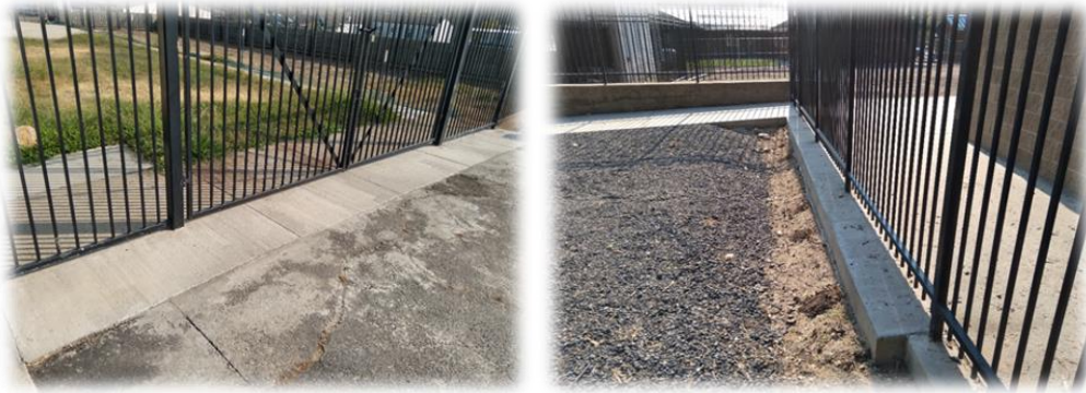
Concrete bases poured for fencing at the Twain Harte and Columbia pools.
