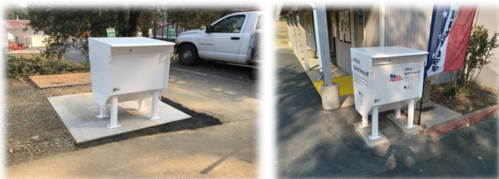
Concrete pads poured for several ballot drop boxes and helped install drop boxes.
